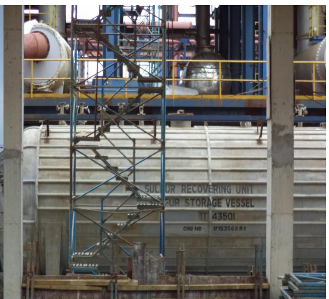
Sulphur Recovery installed at ByProduct plant
