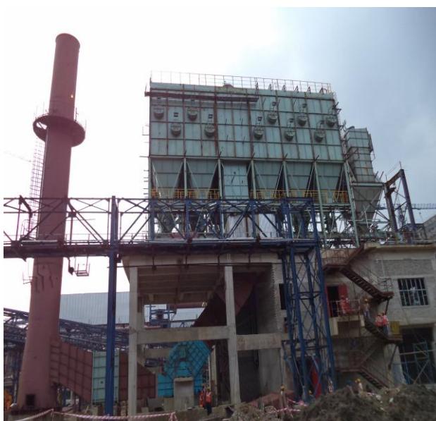
Bag Filter installed for Coke Oven Charging Car
